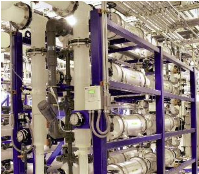
Oxygen removal system
