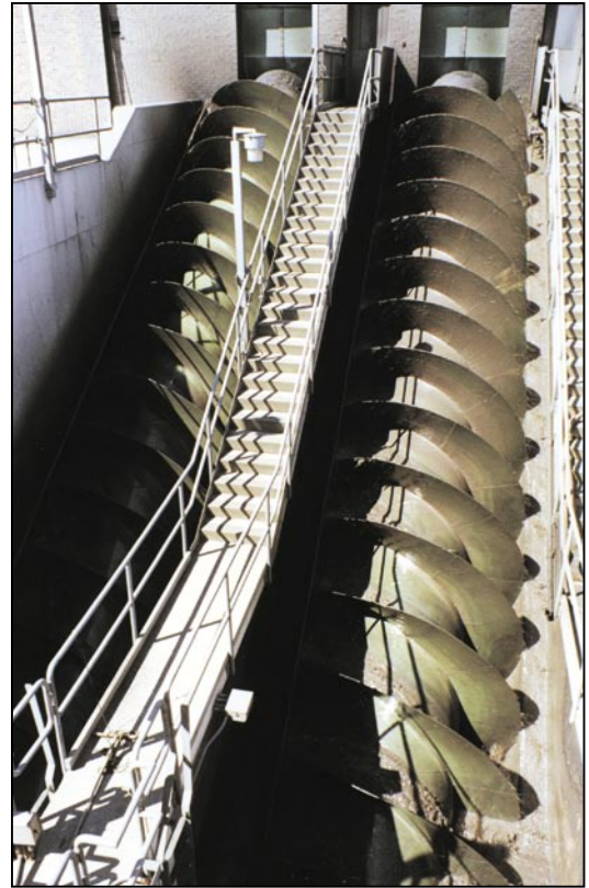
FIGURE 5. Archimedes screw pumps are good choices for delivering raw wastewater to API separators' aboveground tanks
