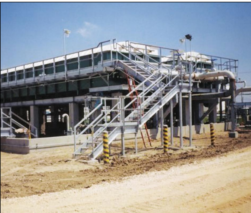
FIGURE 2. For wastewaters containing substances that are toxic or otherwise hazardous, it is prudent to specify steel tanks that are above-ground. This approach also facilitates maintenance and inspection
