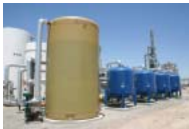
As part of the refinery's boiler feed water system, USFilter provided four multi-media filters to remove suspended solids from groundwater treated at the refinery. Each filter is 84" diameter x 60" side shell, designed for 300 gpm.
