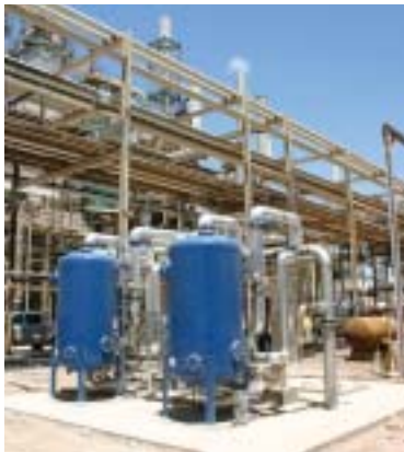
USFilter provided three softeners rated for 300 gpm each for polishing the effluent from the RO system.
