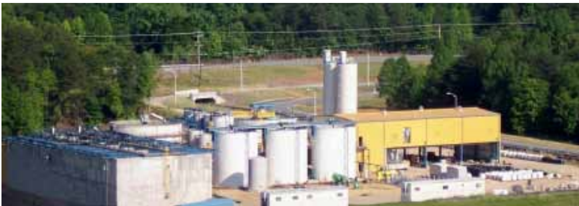
Figure 6: Belews Creek WWTS
