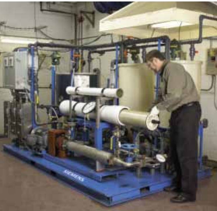
The Membrane Care SM Program provides services to keep systems operating at peak performance.
