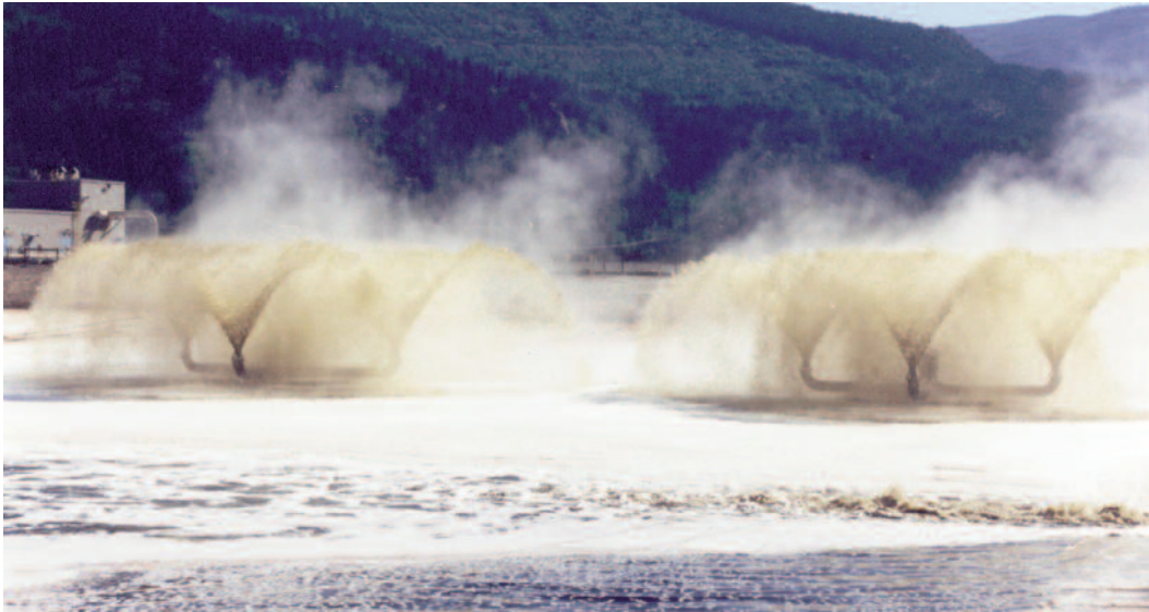
Four-nozzle spray coolers installed at pulp mill
