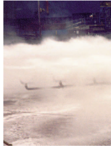
Twelve-nozzle spray coolers installed at steel mill
