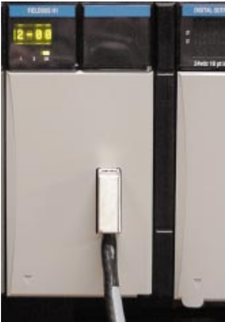
Figure 2 - Fieldbus Interface Module (FIM) mounted in I/O rack
