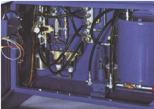
Manual backup closure system housed in enclosed cabinet.
