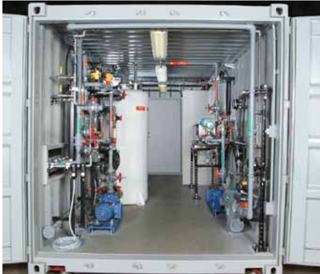
Containerized SiCURE™ system
