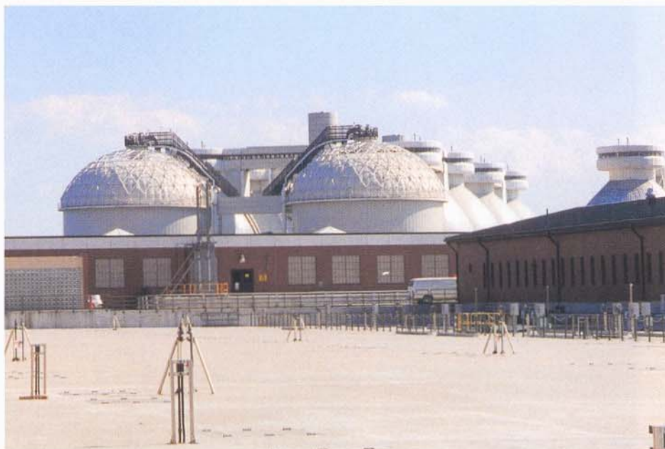
PFT-Dystor® gas holders front the digesters.
