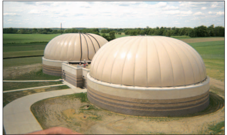
Figure 3: USFilter's anaerobic digestion retrofit program and its Dystor dual membrane gas holder cover (pictured above) are two solutions to digester gas storage.
