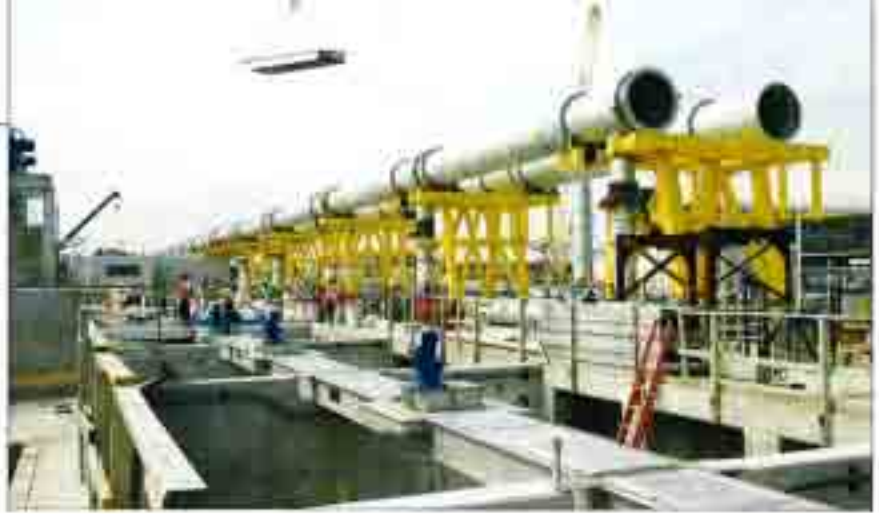
▲ Bridging. Odor control and process air piping spanning aerators required extensive support.
