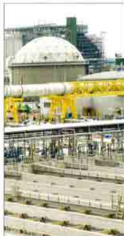
▲ Challenging. Tight site squeezes in old and new digesters and new final sedimentation tanks.
