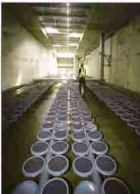
▲ Air. Diffusers will aerate secondary flows.
