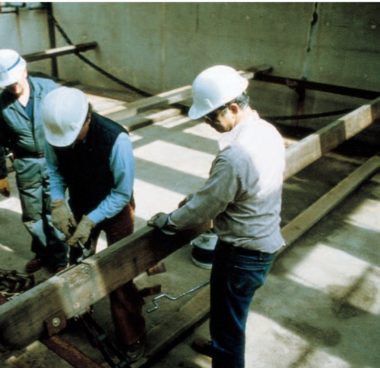
Service personnel remove redwood flights in preparation for installing new fiberglass flights.
