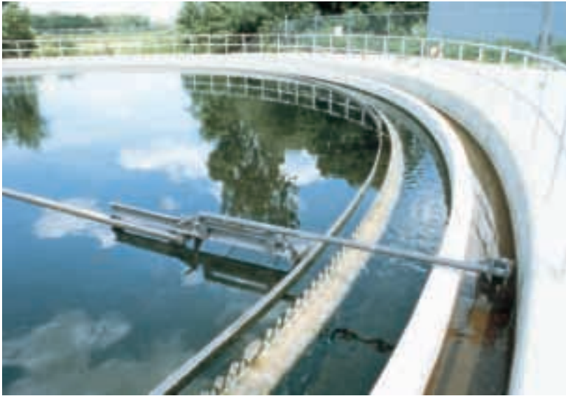
High strength dairy wastes in the effluent do not affect the performance of these two 80-foot diameter Rim-Flo® tanks. Average raw flow is 400 GPD per square foot of overflow. BOD and SS in the effluent average between 3 to 5 ppm.
