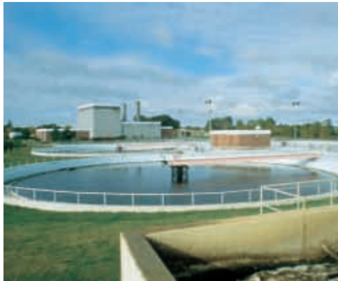
Four 120-foot diameter Rim-Flo® tanks operate at 700 GPD per square foot of overflow in this installation. Effluent quality is 3 to 7 ppm BOD and SS.
