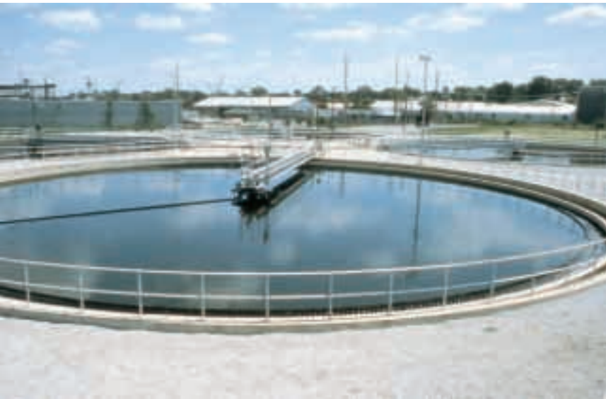
Four 110-foot diameter tanks in this wastewater treatment plant operate at an average raw flow of 400 GPD per square foot of overflow. Effluent BOD ranges from 4 to 6 ppm.
