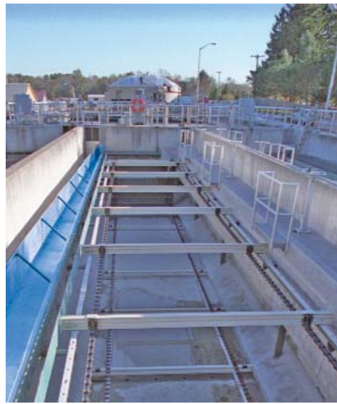
Trans-Flo® clarifier steel trough retrofit in progress. Influent channel and orifices (grey). Effluent channel and weir (blue).
