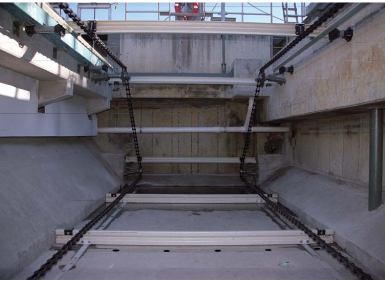
Sludge removal header and orifices (black)
