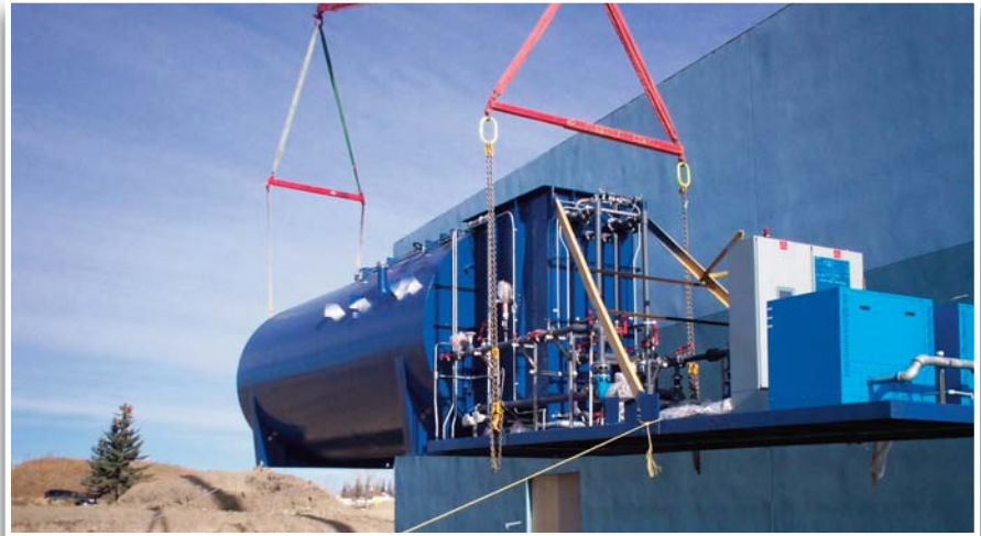
Installation at Grey Eagle Casino in Calgary.
