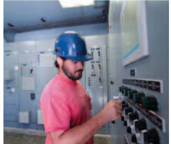
SmartBNR™ Controls provides an efficient operating wastewater treatment facility.
