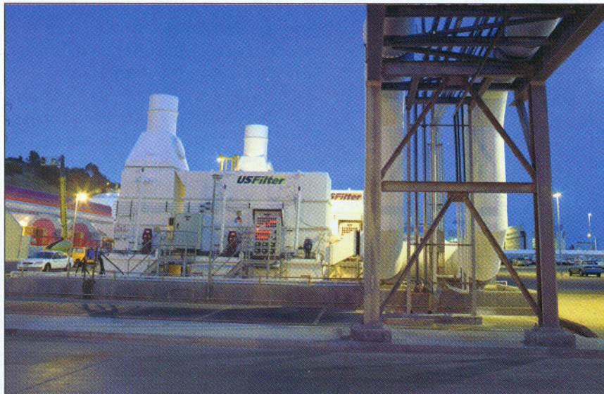
The Hyperion plant is one of the largest in the United States, serving about 4 million people in the Los Angeles area.
