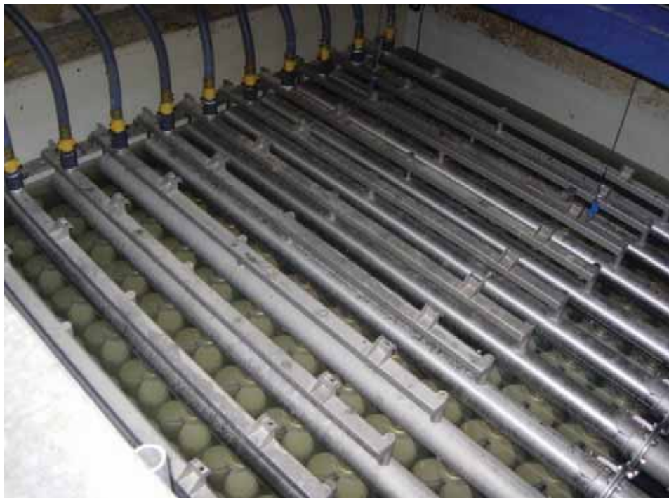
Shown above are the membrane modules installed in the treatment tank.
