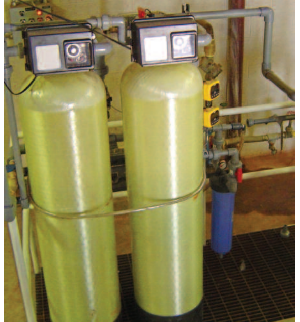
16" diameter automatic, arsenic units
