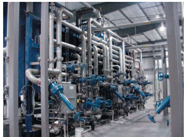
Ion Exchange removal tanks with valves and piping harness for one of two installed systems
