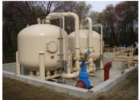
Ion exchange vessels treating 1500 gpm
