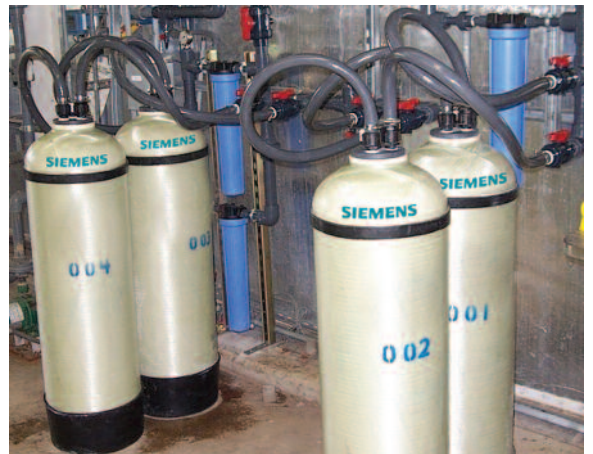
Service Ion Exchange vessels in a lead/lag configuration
