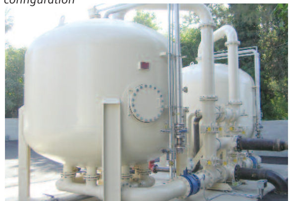
Typical HF1220 tanks operated in a lead/lag configuration
