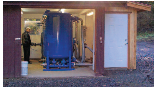
48" carbon steel vessels containing arsenic removal resin
