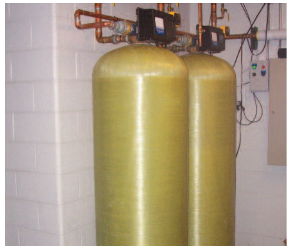
24" diameter duplex vessels treating 50 gpm
