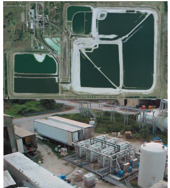
Top: Aerial photo of 540 acre site Bottom: Partial view of equipment. Total includes: (7) trailers, (6) skids and (8) vessels.
