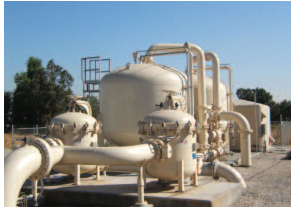
12' diameter Hi-Flow vessels in lead/lag configuration
