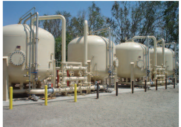
Two trains of HP® 1220 low-flow carbon adsorbers in a lead/lag formation treating 2000 gpm.
