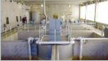
12 MGD (45MI/d) MULTIWASH CentROL Installation
