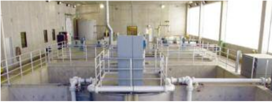
Compact 21 MGD (79 MI/d) CentROL Installation
