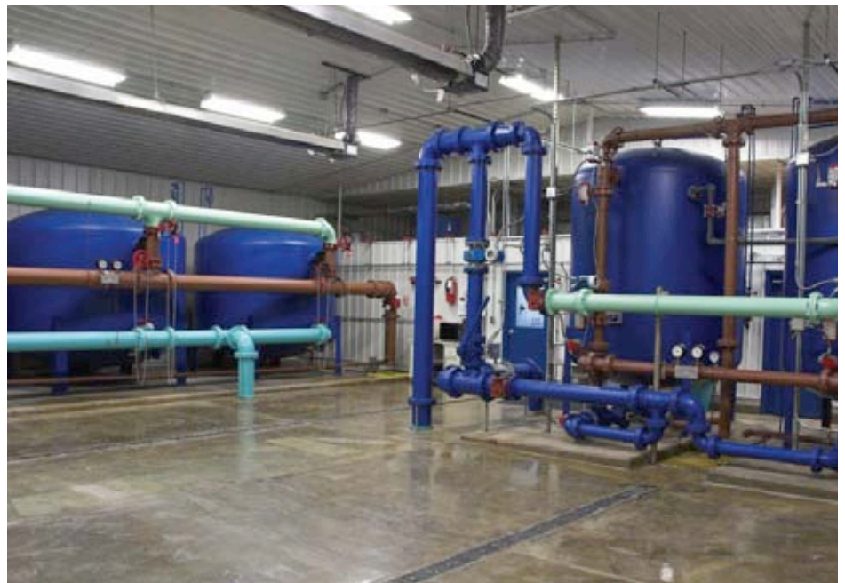
Vertical pressure filters and softeners
