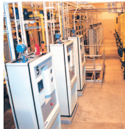
USFilter supplied the largest chlorination-dechlorination system in America.
