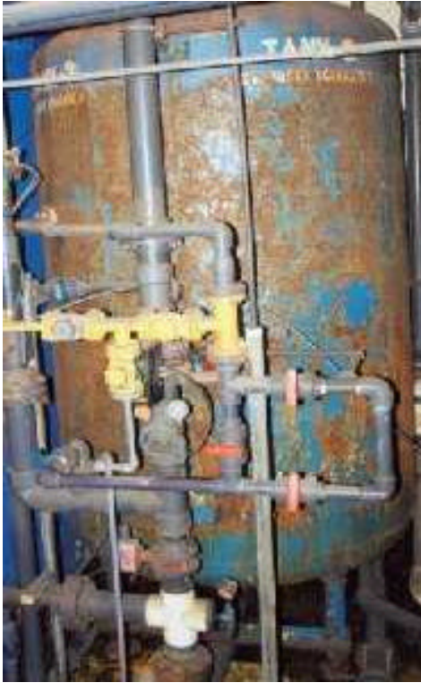
This system is a safety hazard, requires constant operator attention and may fail at anytime. It could shut down production and possibly cause serious harm to workers.
