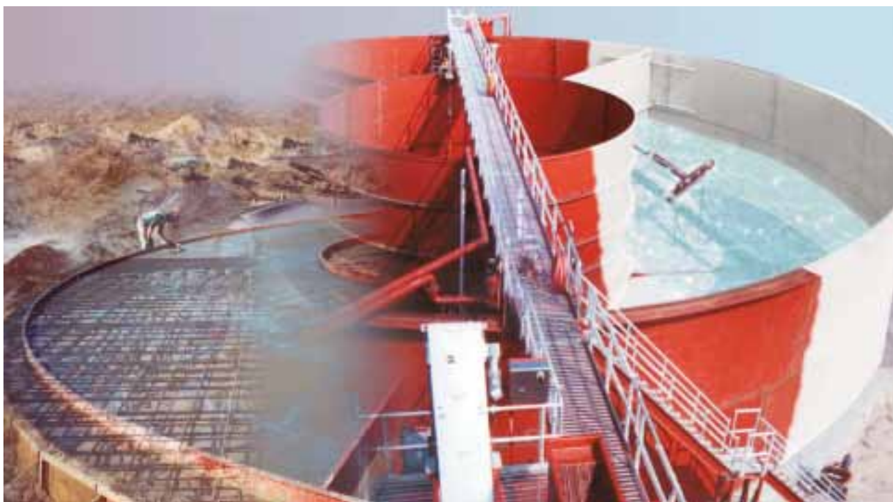
The Sequencing Batch Reactor (SBR) treatment process is ideally suited for biological nutrient removal applications, and those applications requiring high quality effluent at widely varying flows and loadings. These field-erected SBR systems are especially attractive where tight budget constraints and critical scheduling pressures are dominant factors.
