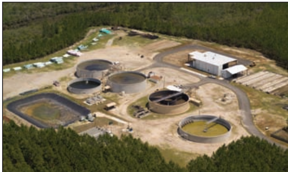
Aerial views of the Point Washington Wastewater Treatment Plant (top), the Sandestin plant (center), and the Seacrest facility.
