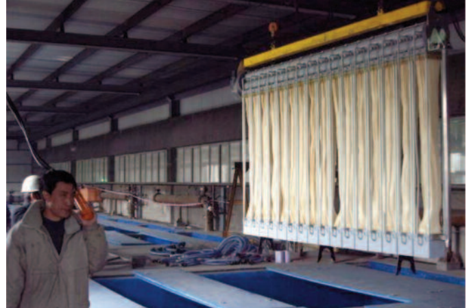
Membrane rack being loaded to an MOS cell
