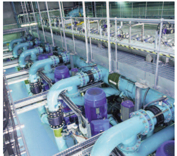
6 cells each contain 192 filtration modules
