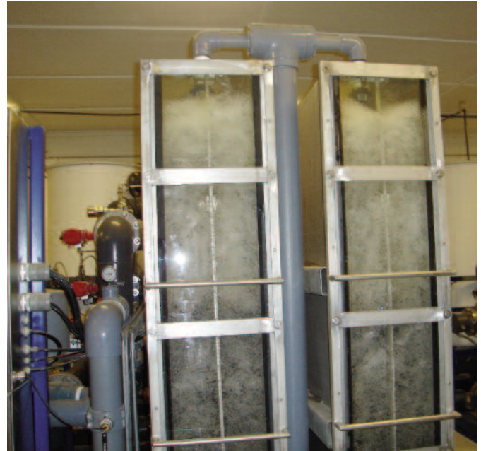
Memcor XS 48 system in backwash cycle.
