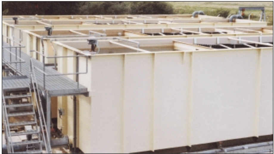
This 4.75 MGD Aquarius plant is located on the Isle of Wight off the coast of England.
