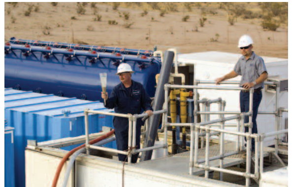
Mobile clarification provided a temporary solution to a weather related condition
