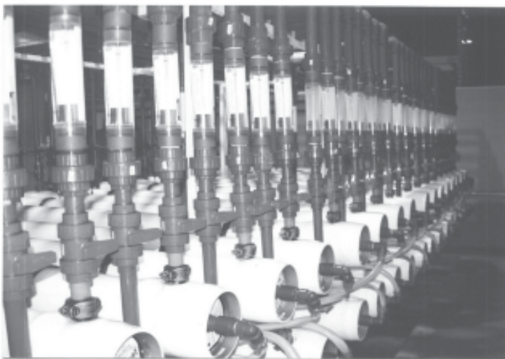
Figure 1. Off-site cleaning skid.
