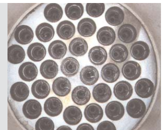
Cyclone clarifiers inside the vessel.
