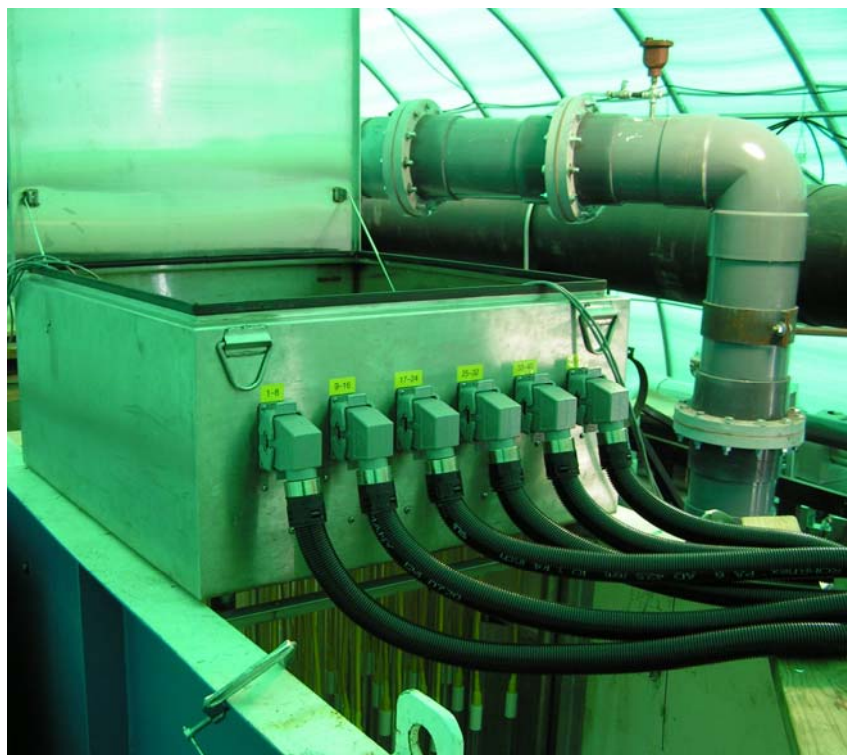
Figure 3. Photo of the Installed Barrier Sunlight V-48E-A300 in Validation Test Channel
