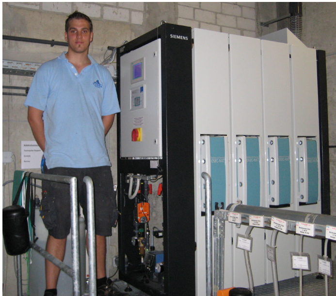
Center's technician, Florian Egner, stands next to installed membrane electrochlorination system.
