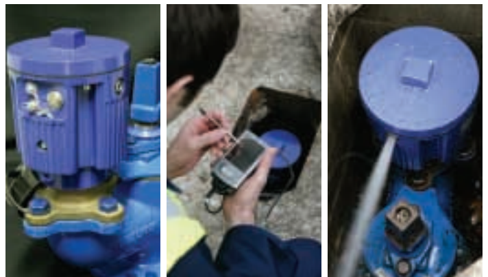
HydraClam ® water quality monitor fitted to standard hydrant
