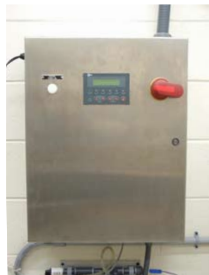
PLC based control panel
