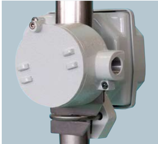
Electronic Flow Transmitter mounted on meter body
