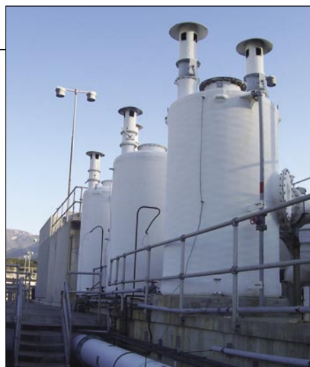
Three Midas odor control towers at a wastewater treatment plant in Las Virgenes, Calif.
