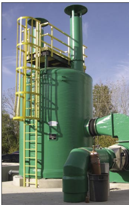
USFilter's Midas odor-control activated carbon is the filling for this adsorption tower in Columbus, Ohio
