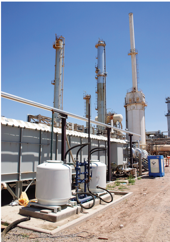
FIG. 2 Activated carbon remains a cost-effective treatment technology for air, water and process purification.
