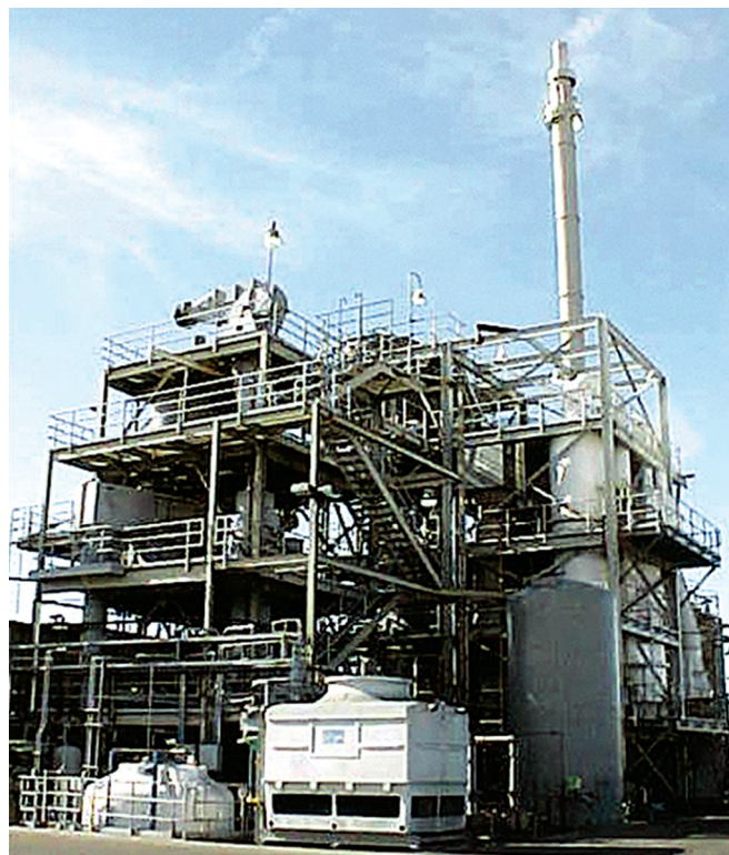
FIG. 1 Multiple Hearth furnace plant in Parker, Arizona.
