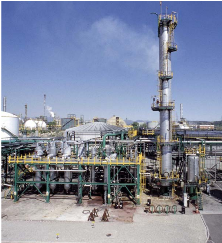
Figure 3. Wet oxidation system. Feed effluent heat exchangers on left, reactor on right, phase separator on far right.
