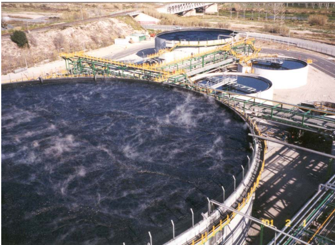
Figure 7. Repsol PACT® system. Tanks (clockwise from lower left), PACT-1 aeration tank, PACT-2 clarifier, PACT-2 aeration tank (top), PACT-1 clarifier, spent carbon feed tank (far right), and sludge thickener (center). Note black color of liquor, due to the powdered carbon.
