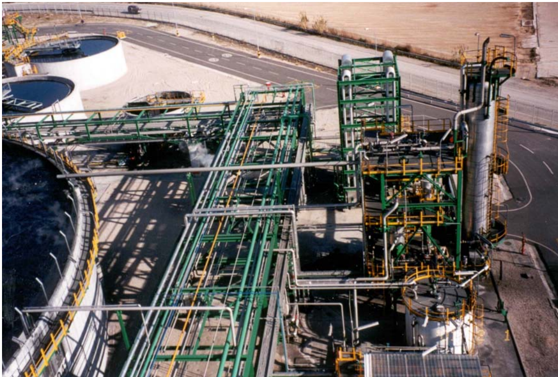
Figure 9. Repsol WAR system. PACT® system on far left. Sludge feed tank on left (back), vertical U-bend heat exchangers in back, WAR reactor on far right. WAR system ash blowdown tank (right corner) for feeding the filter press.
